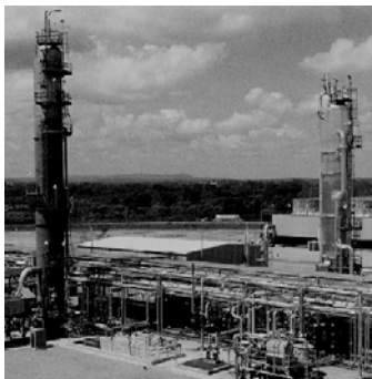
Fig. 2a. An amine-based post-combustion CO 2 capture system treating a portion of the flue gas (~40 MW equivalent) from a coal-fired power plant in Oklahoma, USA. (Photo courtesy of U.S. Department of Energy)
